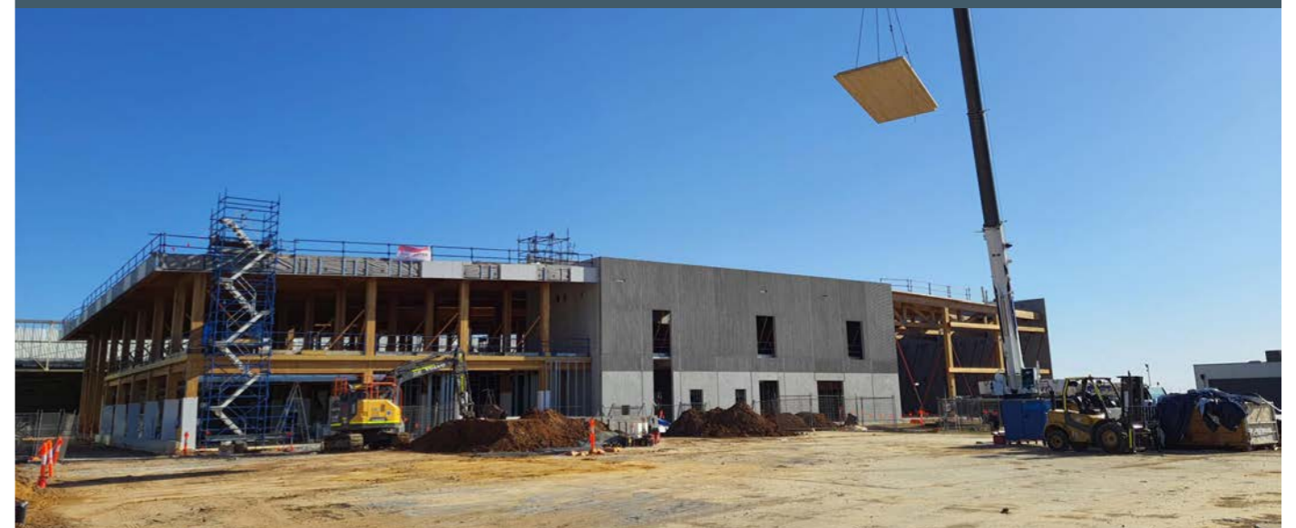
A crane hoists a NeXTimber CLT panel used in the construction of the building.
