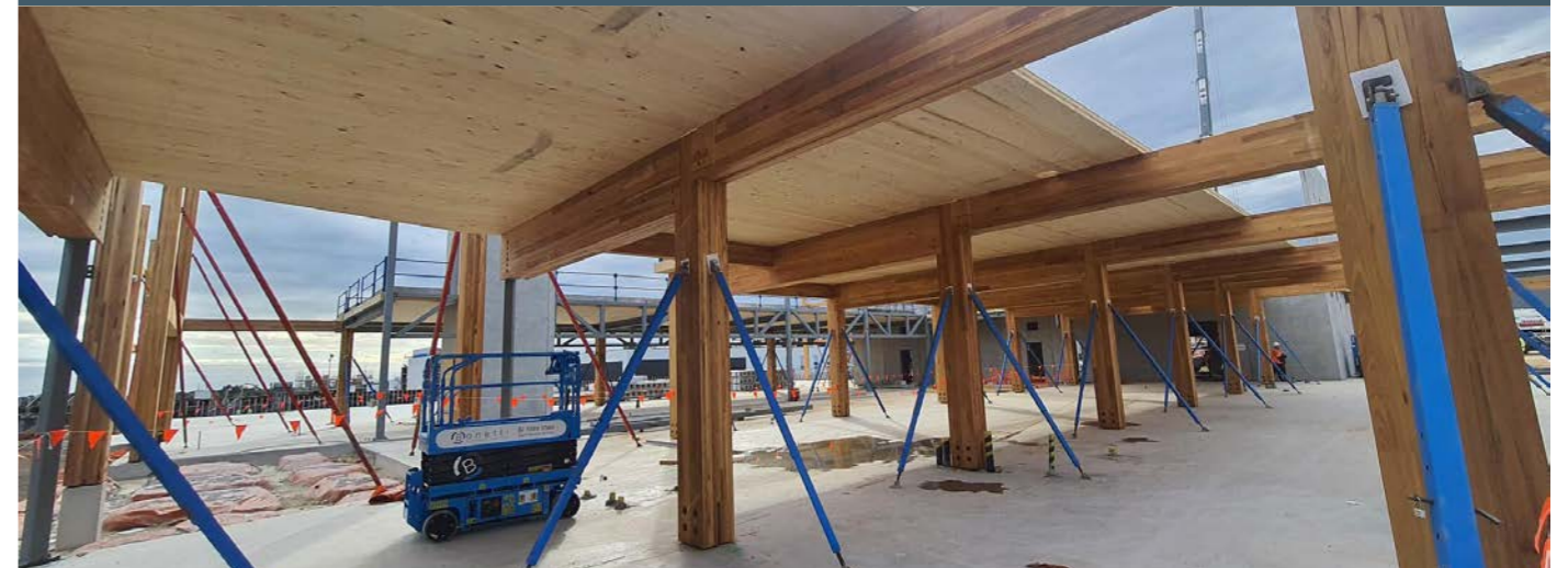
NeXTimber prepared the draft documentation based on the technical information provided by the customer including 3D modelling of the CLT structure, the loading drawings, shop drawings of the individual CLT panels and the assembly sequence drawings.
